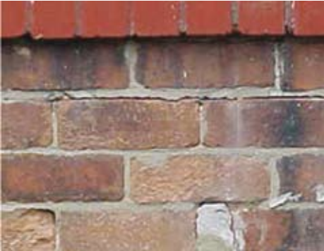
Fig 4 - Horizontal cracking in mortar joint
