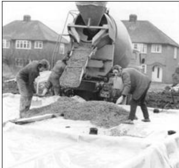
Figure 4: Laying of concrete in the mid 1970s on a 300 micron damp-proof membrane that has been placed over hardcore in the foundations of a house.
