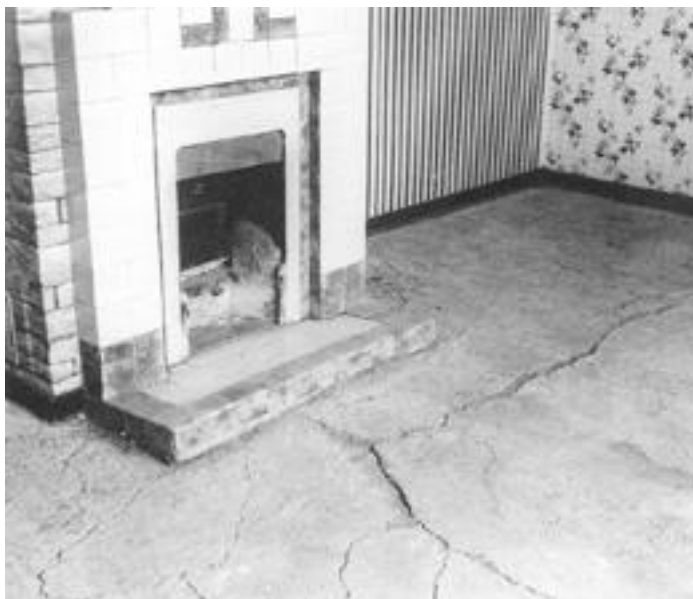
Figure 1: Distortion and cracking of a concrete floor slab caused by sulfate attack. Damage is greatest in front of the fireplace where water, carrying sulfates from underlying hardcore, has been drawn through the slab by heat from the fire.
